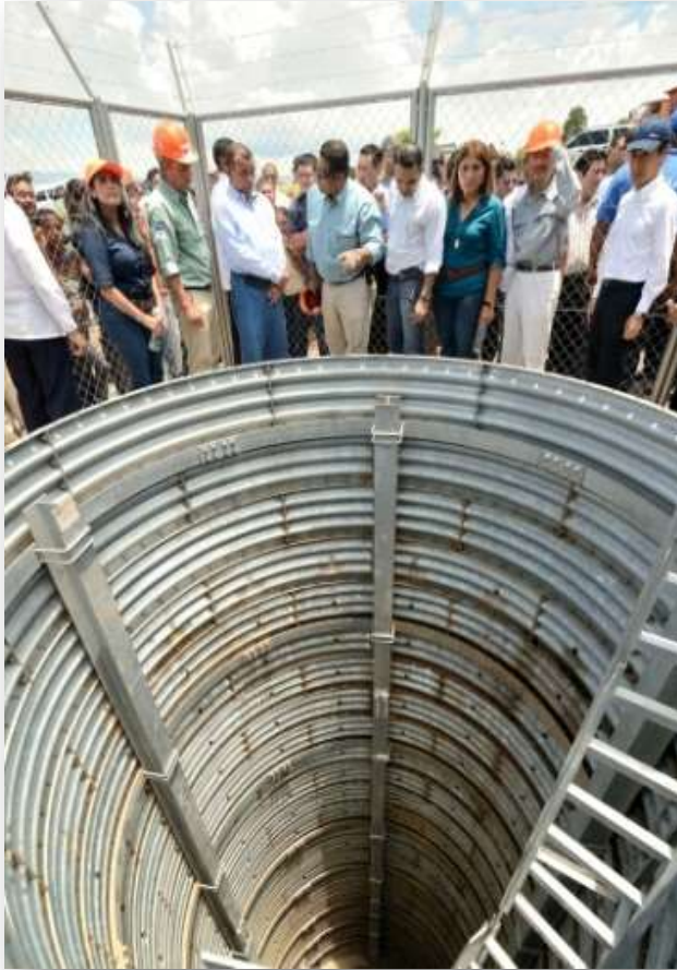
Drainage well in Honduras
