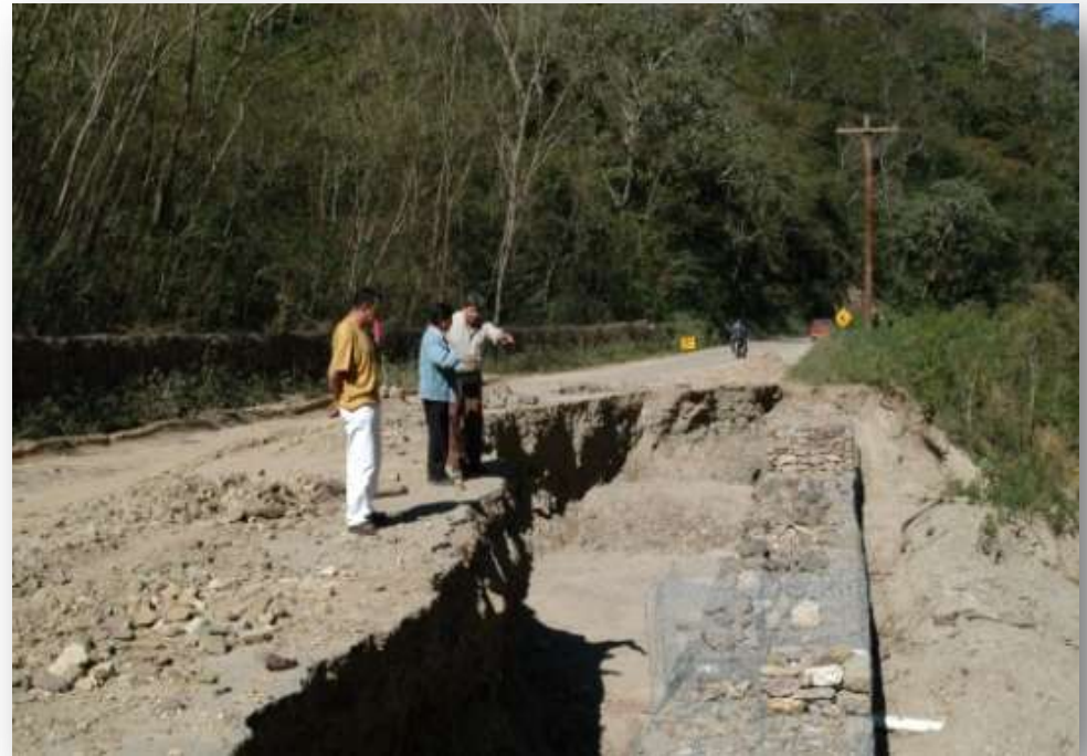
Damage on Route 7 after a landslide (Bolivia)
